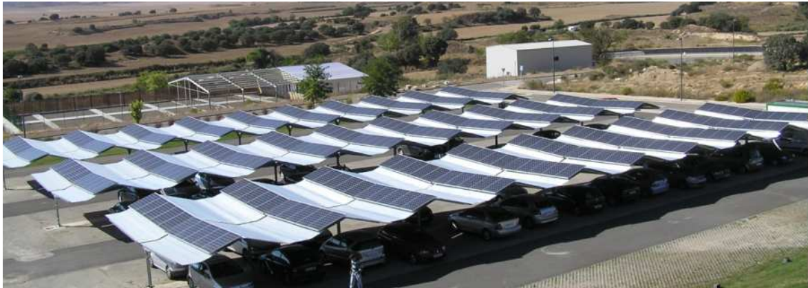
Fig. 1.3. Fixed installation in parking canopies of Walqa Technological Park.
