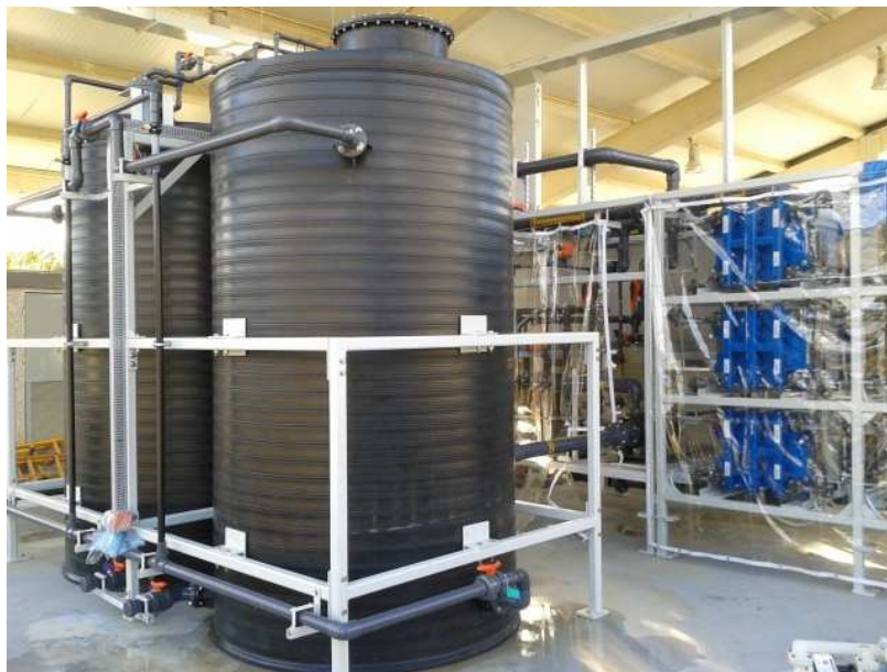
Fig. 4.2. View of the tanks (left) and the stacks (right) of the flow battery
