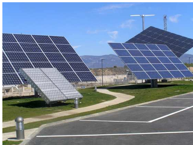
Fig. 2.4. DEGUER solar trackers and behind MECASOLAR solar tracker.
