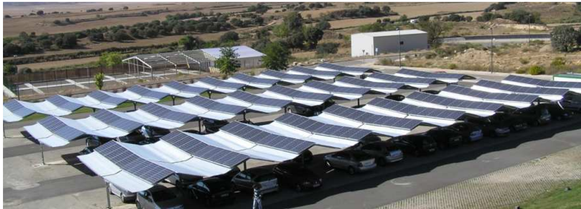
Fig. 2.3. Fixed installation in parking canopies of Walqa Technological Park.
